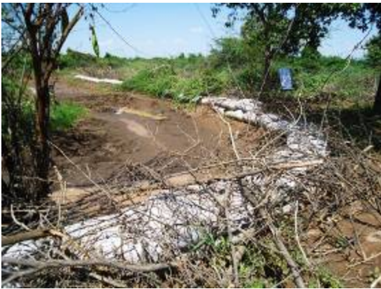
Figure 16. The dam's embankment built with “Do-nou” covered with the branches of Acacia
